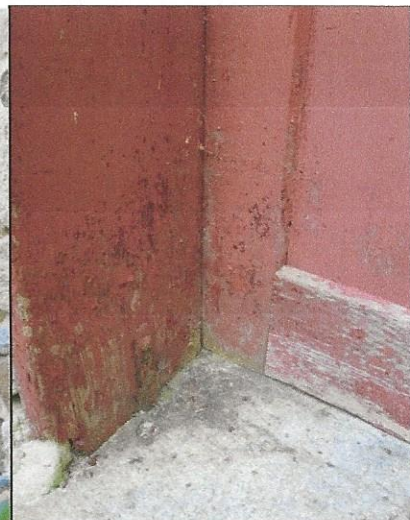
(Rotten doors and frames)
