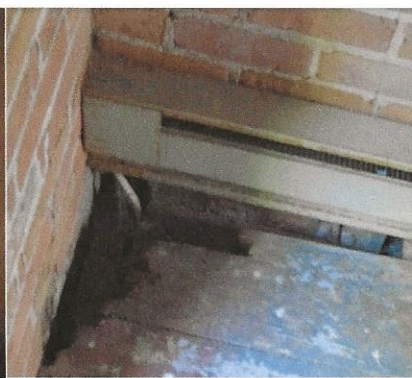
(Holes in floor)
