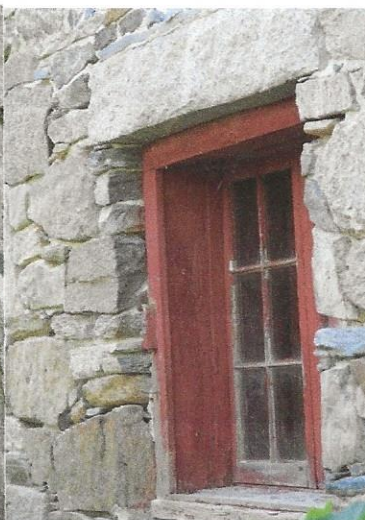
(Rotten sills and trim)
